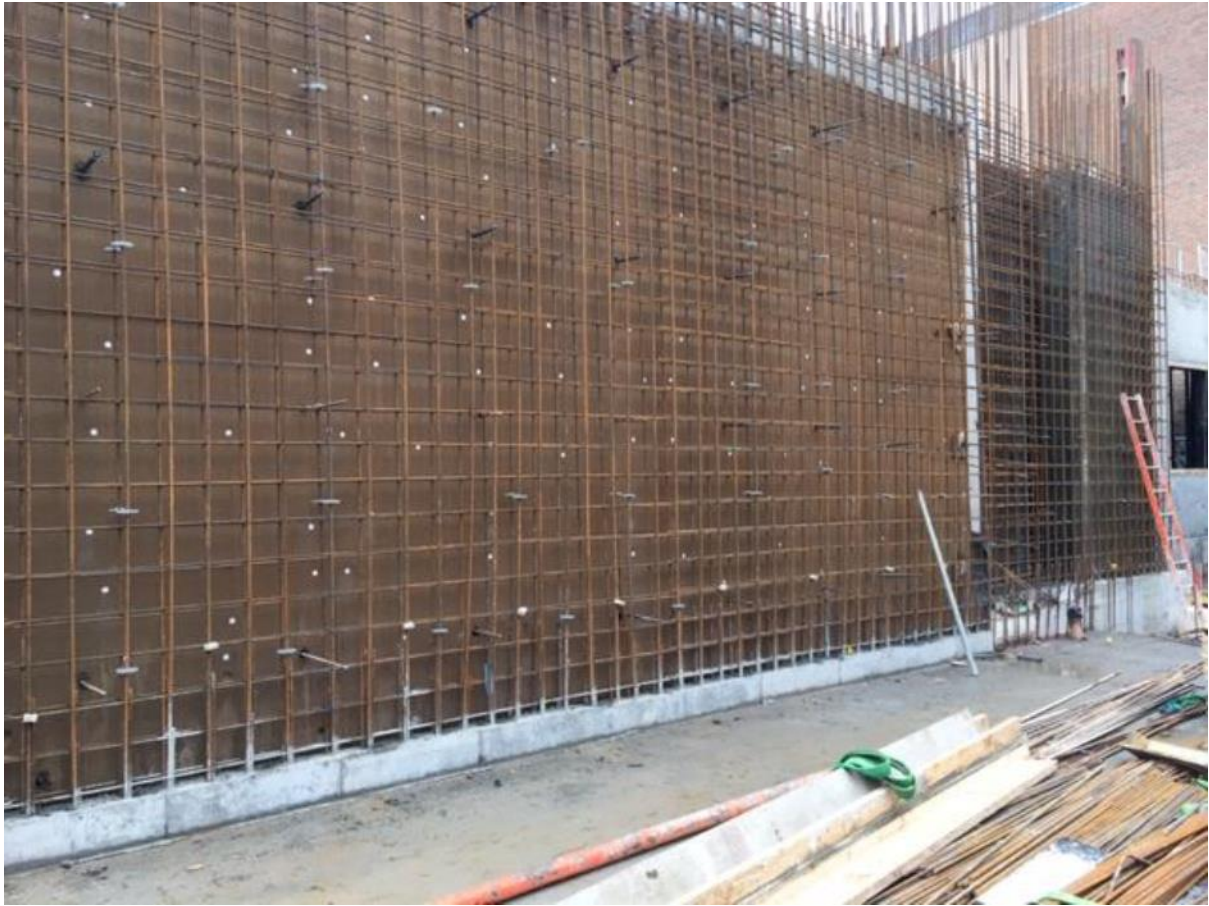
Ground – 1st Floor walls been cast at GL 25b in Corner Building
